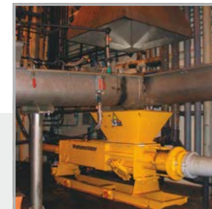
Pumping screenings (Coney Island, New York)
