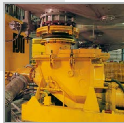
Above: Coal sludge reception system in a power plant Below: KOS 2180 coal transportation pump for longdistance coal delivery
