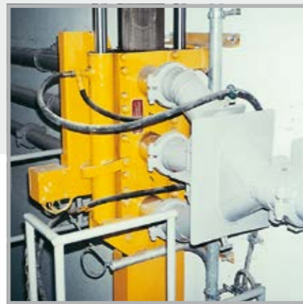
Gate valves for there different delivery lines
